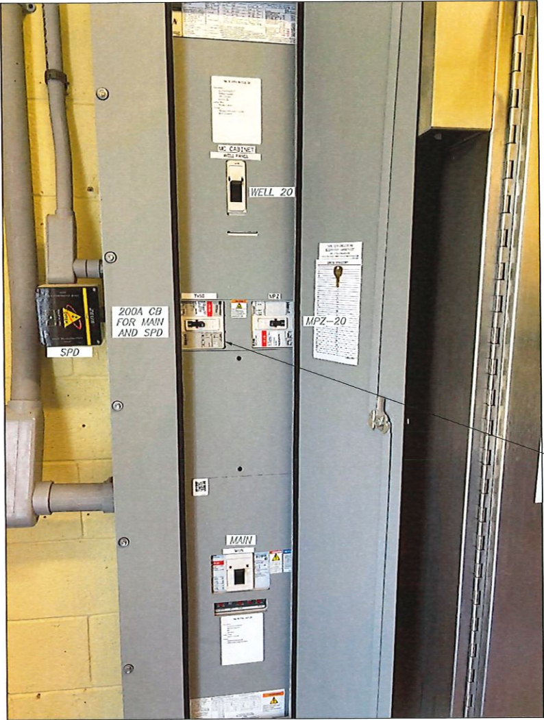
PHOTO 2 EXISTING PANEL HP-20 MFG: EATON POW-R-LINE SERIES EATON JOB NO: STA1058477-001 RATINGS: 400A, 480V, 3PH, 3W, 35KAIC
