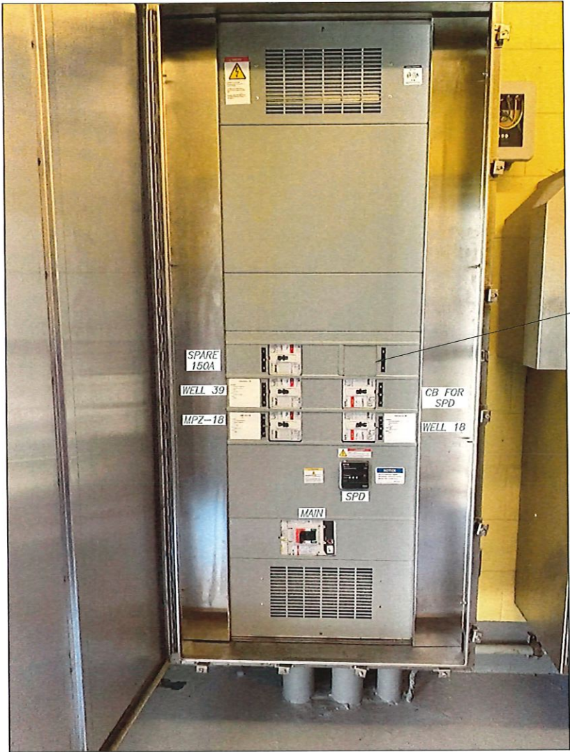
PHOTO 1 EXISTING PANEL HP-18 MFG: EATON POW-R-LINE SERIES EATON JOB NO: VONA0526X0K2-0002 RATINGS: 600A, 480V, 3PH, 3W, 35KAIC
